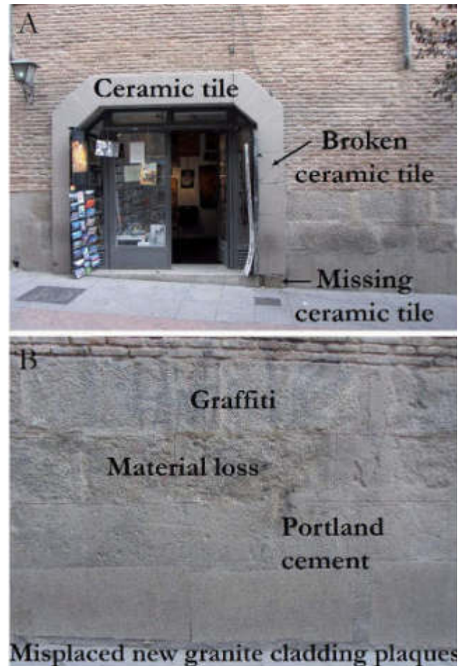
Figure 5.- CTDOSI plinth facing Huertas Street. A: Granite replacement by ceramic tile. B: Anthropic decay in the plinth.
