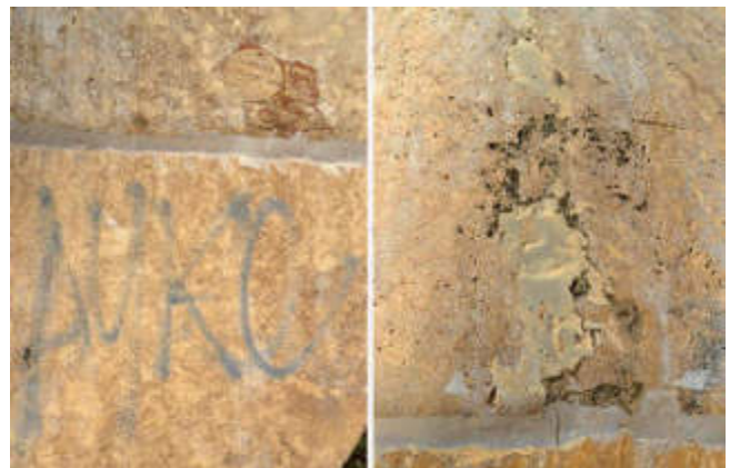
Figure 2.- Miguel Moreno, Luna. Natural stone, monumental proportions. Detail of the work's damage. Source: María del Carmen Bellido.
