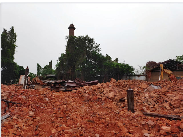
Figure 2.- Surviving Chimney of the now demolished Steam Loco Shed of the East Indian Railways at Allahabad (now Prayagraj). (Photo courtesy Vaibhav Maini)
